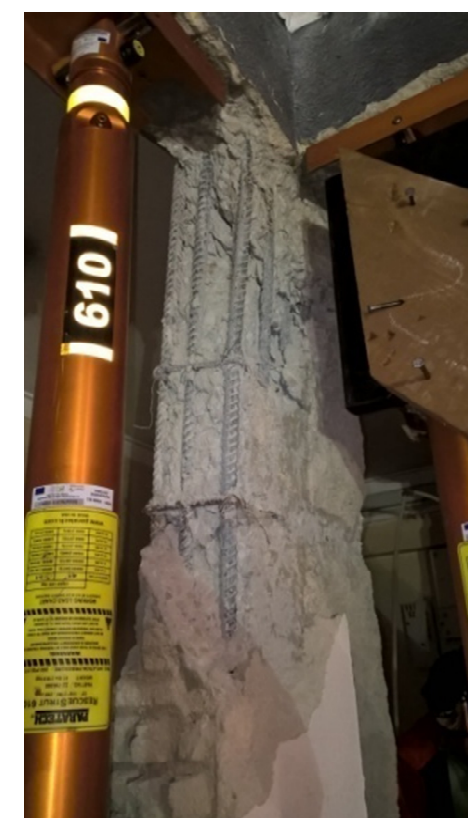
► Fig. 2: Concrete column affected by na explosion
