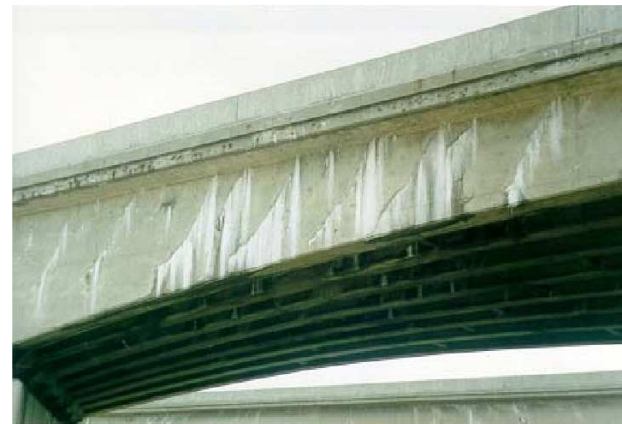
(b) Shear cracks on beam stem
